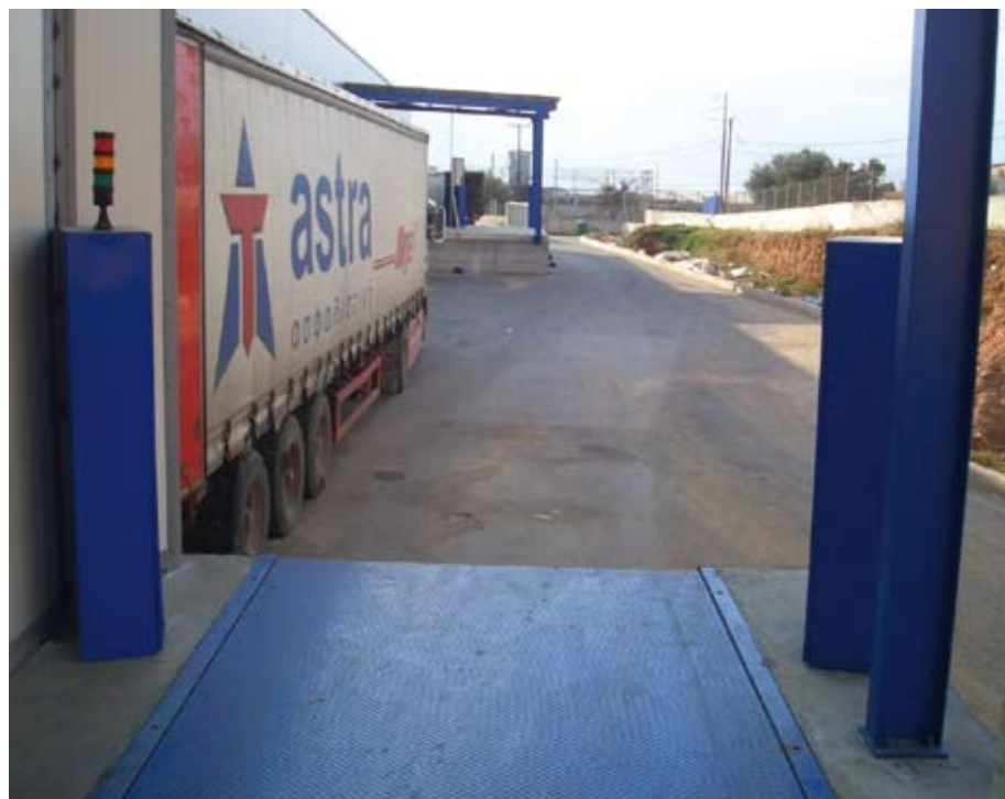
RFID reader portal on the dock doors
